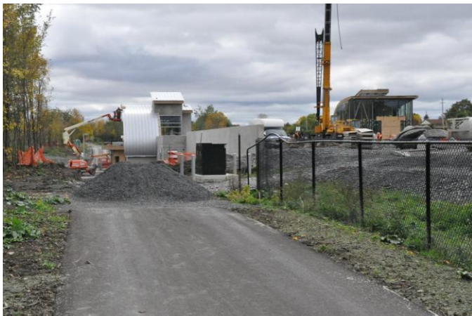
From the Oriska Way end, paved path currently extends as far south as the new Longfields Station, which is seen here under construction. Photo: CfSC
