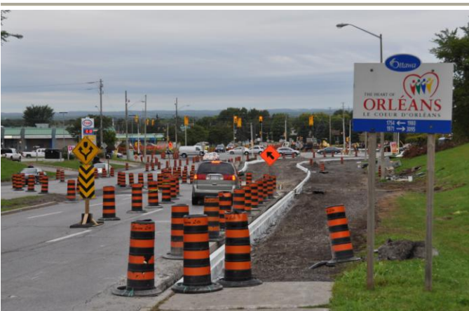
New roundabout takes shape at St Joseph and Jeanne d'Arc in Orleans. This is one construction zone that is not (yet) cycle-friendly. Photo: CfSC
