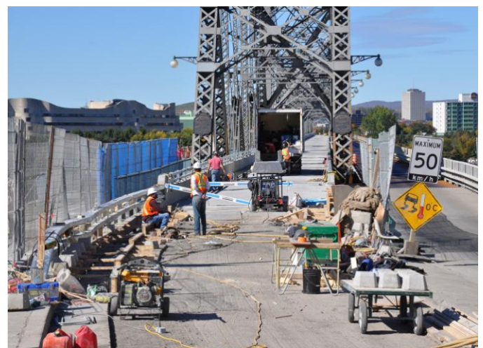
Road construction encroachments on the multi-use path prevented reliable data from being gathered at the Alexandra Bridge CTAP location for much of 2010. Photos: CfSC
